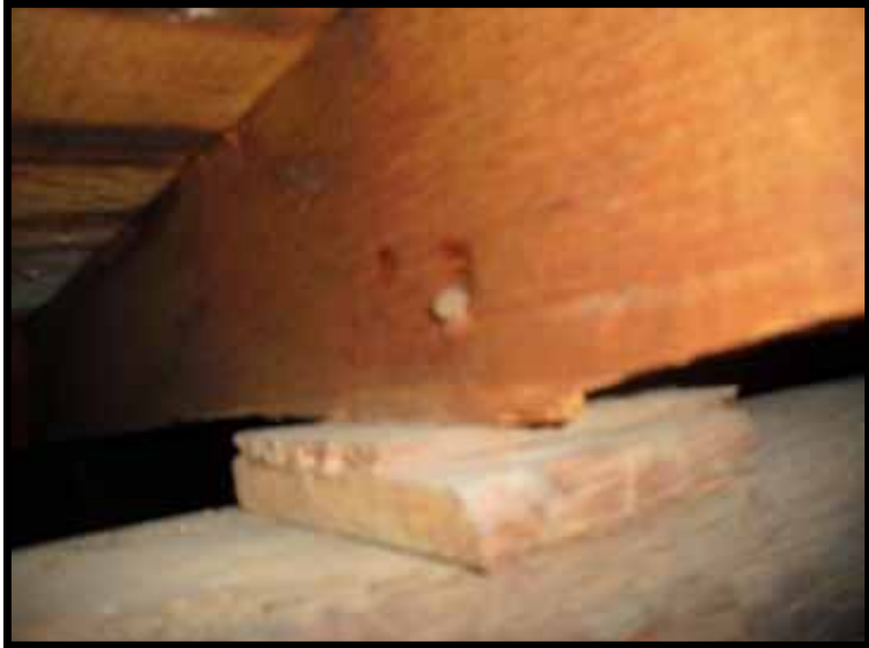
43. TYPICAL ATTACHMENT OF RAFTER TO TOP OF BEAM HAS SHIM PLUS A SINGLE TOE NAIL.
