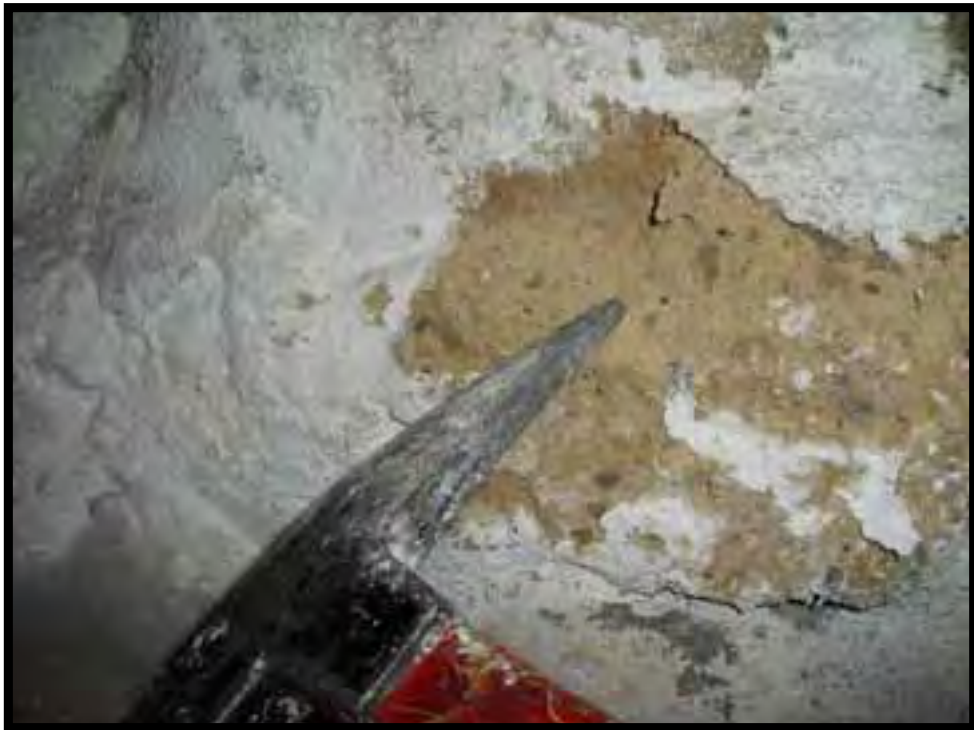
6. QUALITY OF ORIGINAL MORTAR IS LIKE DAMP SAND.
