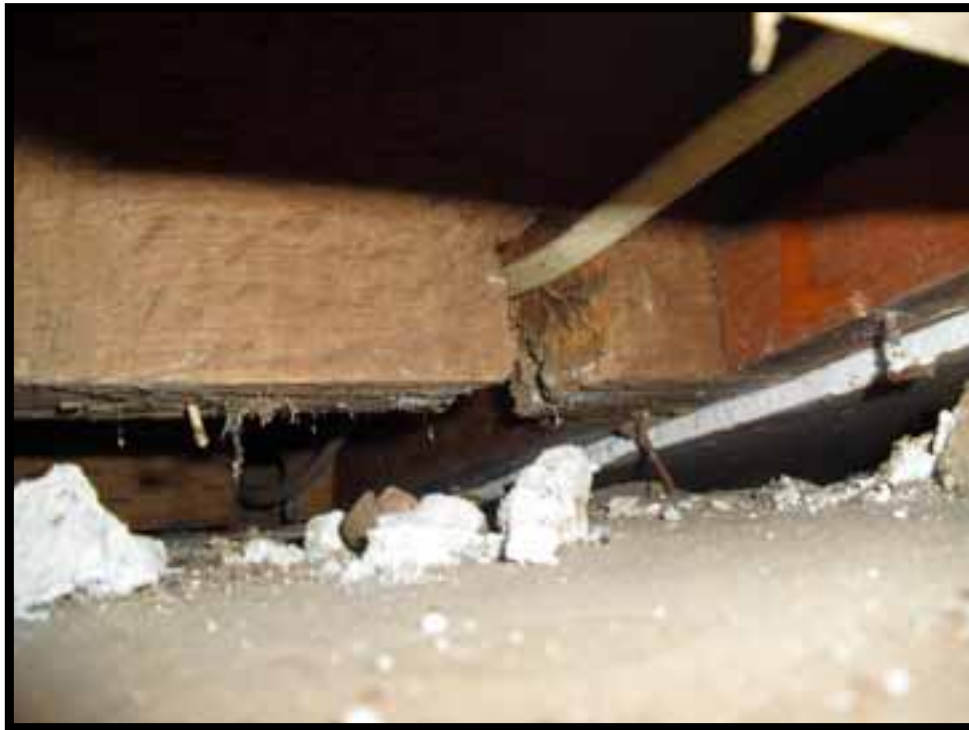
1. 3X10 FIRST FLOOR JOIST NOTCHED NEAR MID-SPAN FOR WIRING.
