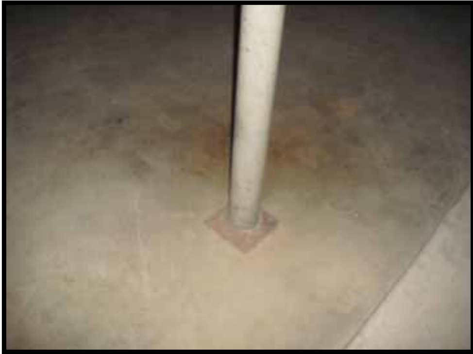
17. COLUMN BASE PLATE AT BEAM SEEN IN PHOTO 16 SITS ON FLOOR SLAB, NOT ON A FOOTING.
