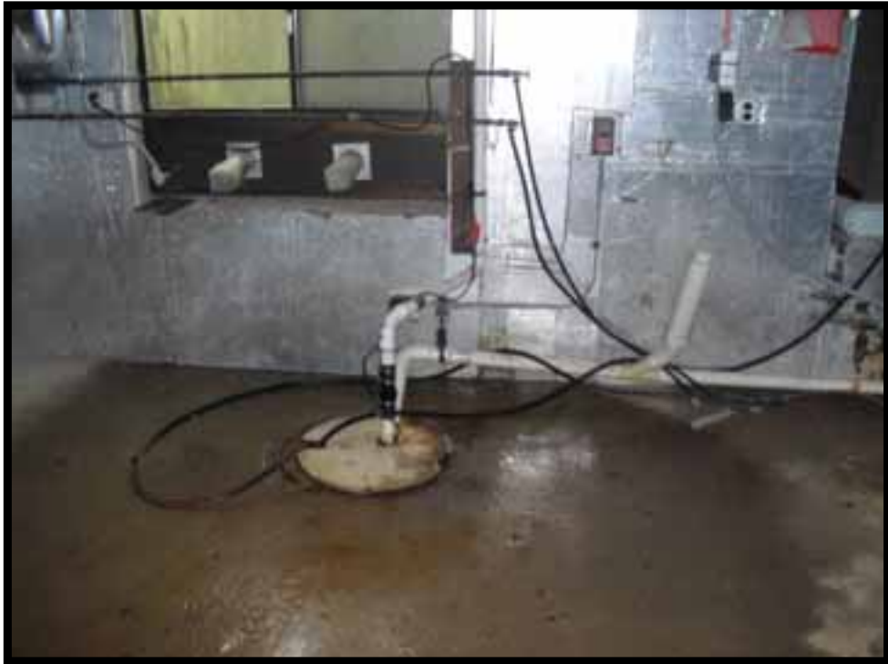
13. DISCONNECTED LINE FROM SUMP SPRAYING WATER IN N-W CORNER BASEMENT ROOM.
