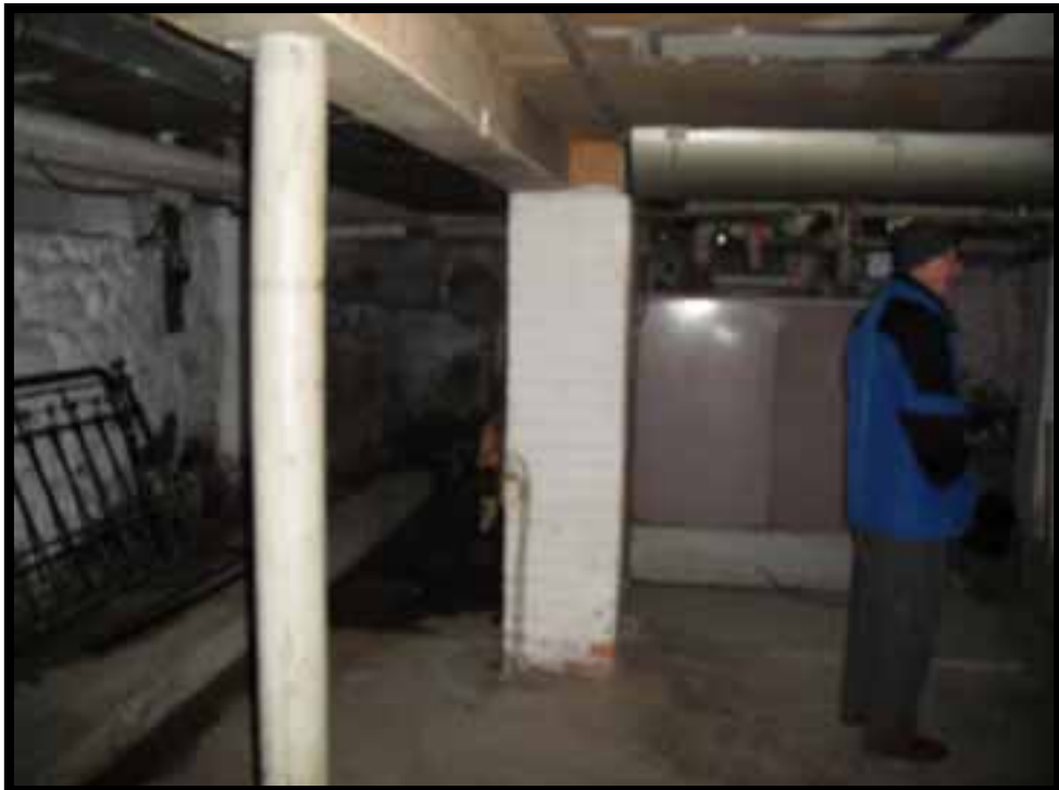
18. PIPE COLUMNS (LIKELY NON ORIGINAL) AND BRICK PIER SUPPORT 8X8 TIMBER BEAM IN BASEMENT.
