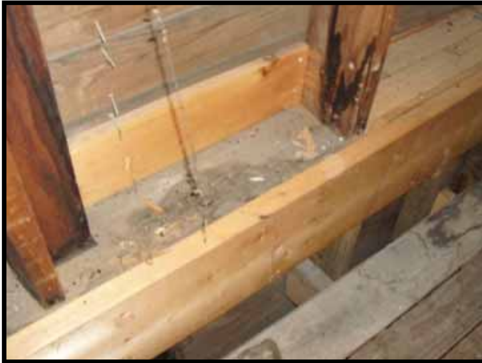
39. EAST GABLE END WALL NEAR ATTIC FLOOR. NOTE: ATTIC FLOOR JOISTS FRAME TO SIDES OF WALL STUDS. IRREGULAR SPACING OF STUDS AND FLOOR JOISTS.
