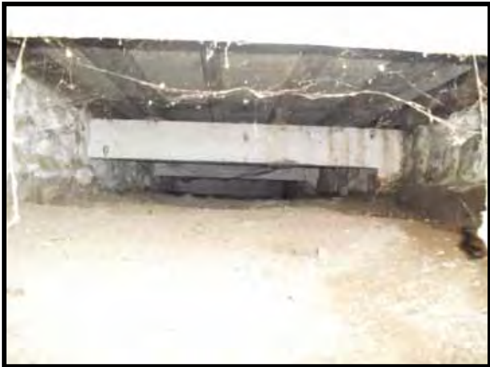
14. CONCRETE BEAMS SUPPORT WOOD FLOOR JOISTS OF THE NORTH PORCH. OTHER PORCHES ARE SIMILAR.
