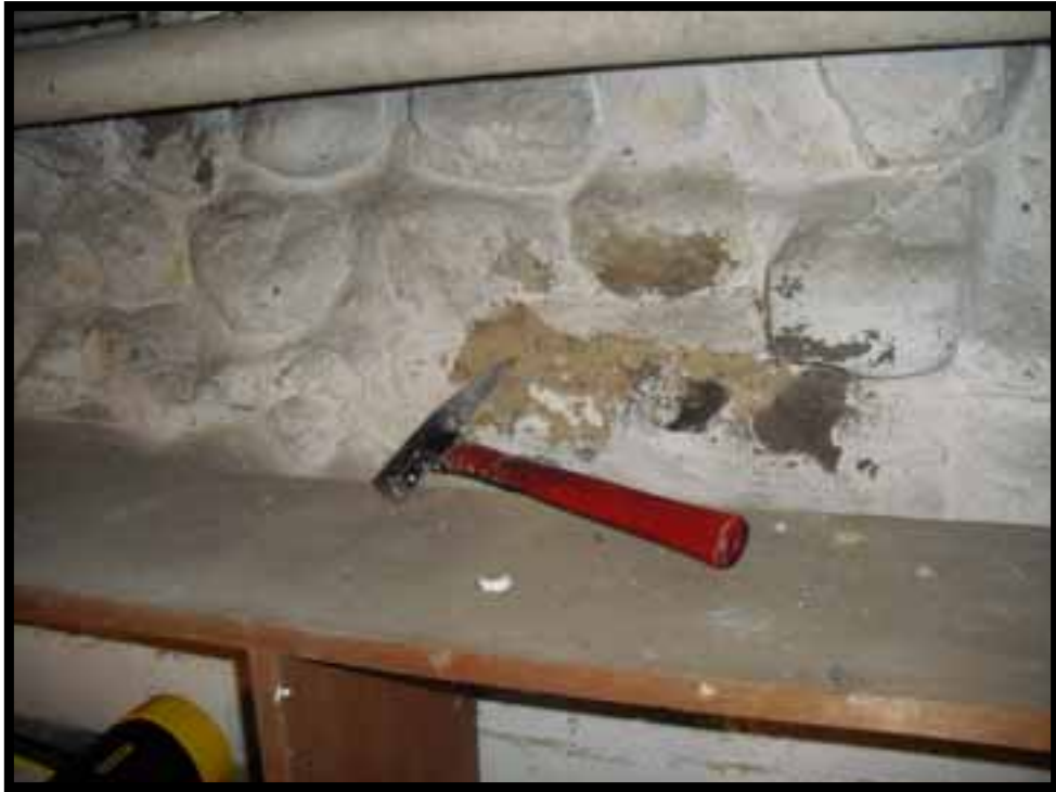
5. QUALITY OF ORIGINAL MORTAR IS LIKE DAMP SAND.
