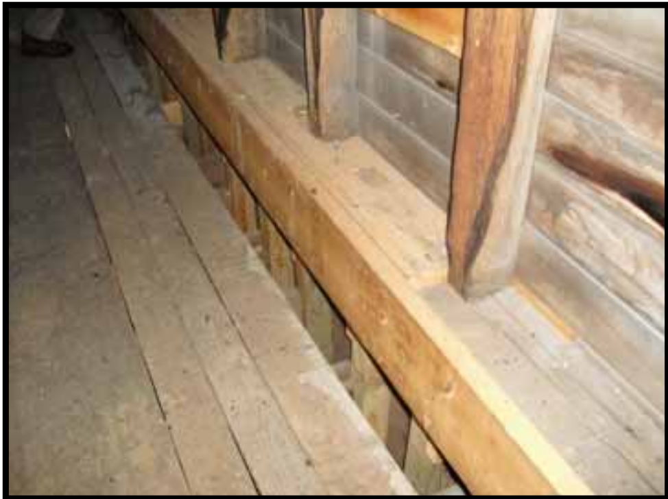
38. EAST GABLE END WALL NEAR ATTIC FLOOR. NOTE: ATTIC FLOOR JOISTS FRAME TO SIDES OF WALL STUDS. IRREGULAR SPACING OF STUDS AND FLOOR JOISTS.
