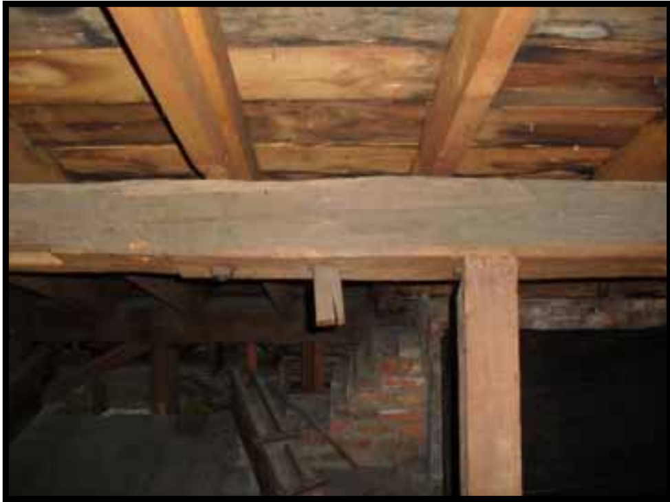
33. LOOKING NORTH AT SCARF JOINT IN TIMBER PURLIN.
