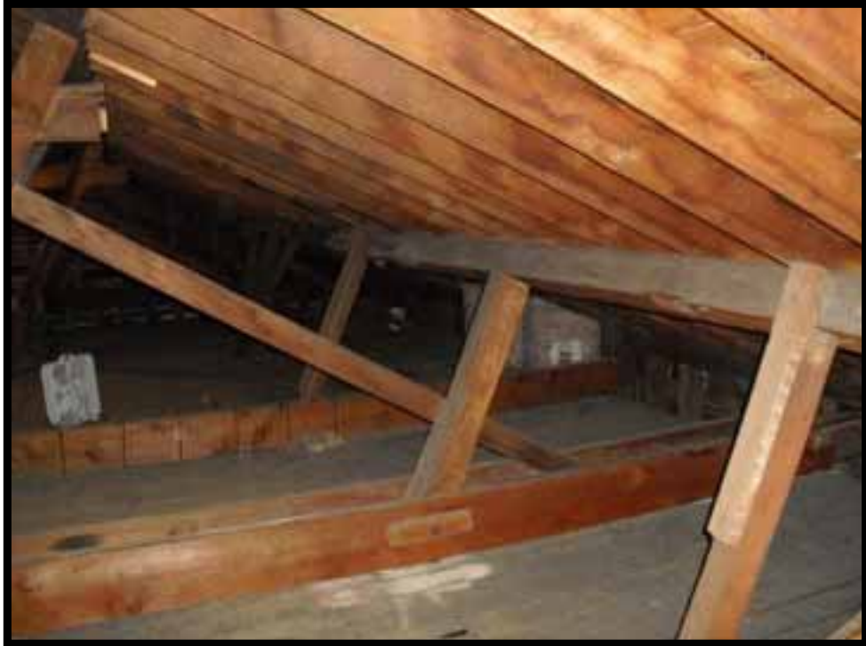
25. ROOF FRAMING LOOKING SOUTH EAST. NOTE NUMEROUS NON ORIGINAL BEAMS ABOVE ATTIC FLOOR SUPPORTING ROOF STRUCTURE AND HANGING ATTIC FLOOR STRUCTURE.
