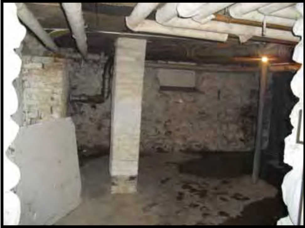
7. SOUTHWEST CORNER BASEMENT ROOM LOOKING SOUTH WEST. NOTE WATER ON FLOOR AROUND CELLAR DOOR.
