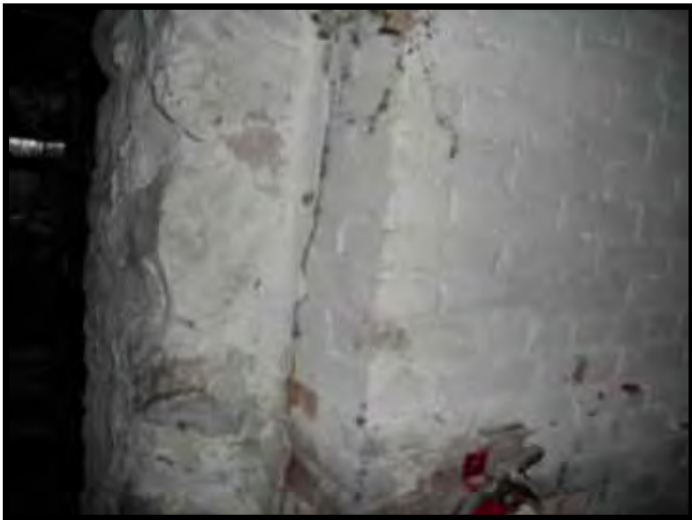
22. CRACK BETWEEN NORTH WEST BRICK CHIMNEY AND STONE FOUNDATION WALL.
