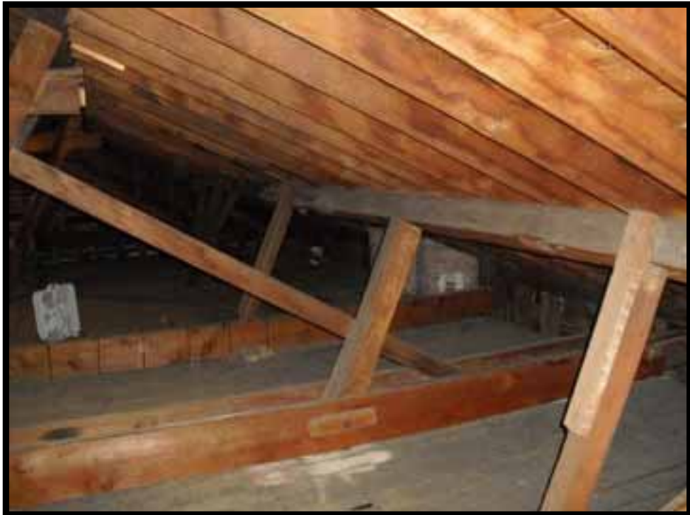
26. ATTIC FLOOR LOOKING EAST. NOT NON ORIGINAL BEAMS ABOVE ATTIC FLOOR SUPPORTING ROOF FRAMING AND HANGING FLOOR FRAMING.
