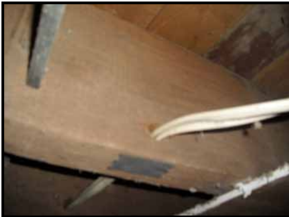
2. 3X10 FIRST FLOOR JOIST WITH HOLES NEAR BOTTOM OF MEMBER NEAR MID-SPAN.
