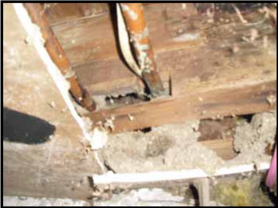
8. PLUMBERS HAVE DAMAGED FIRST FLOOR JOISTS IN SOUTHWEST CORNER ROOM.
