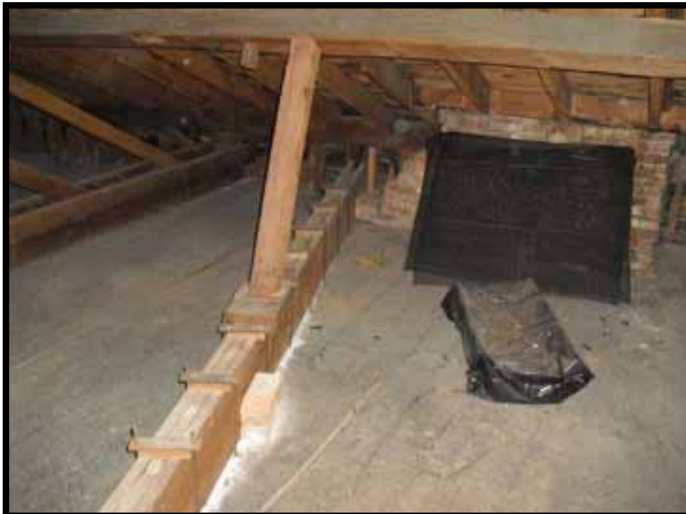
40. NON ORIGINAL FLOOR BEAM ABOVE ATTIC FLOOR HANGS ATTIC FLOOR JOISTS AND SUPPORTS INCLINED COLUMN FROM ROOF PURLIN. THIS IS LOOKING NORTH.
