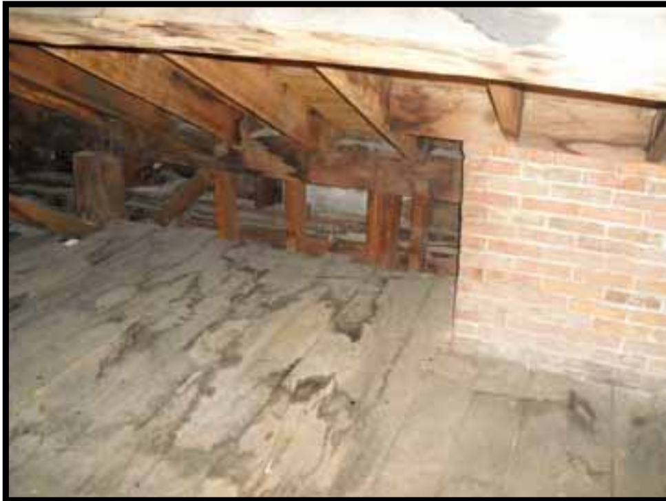
29. ATTIC FLOOR BOARDS AND ROOF FRAMING SHOW EVIDENCE OF PAST WATER LEAKAGE BUT WERE DRY DURING MY INSPECTION.
