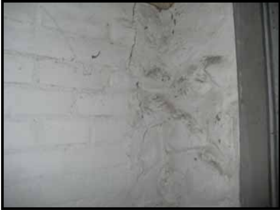
9. CRACKS BETWEEN SOUTHWEST CHIMNEY BRICK AND STONE FOUNDATION WALL.
