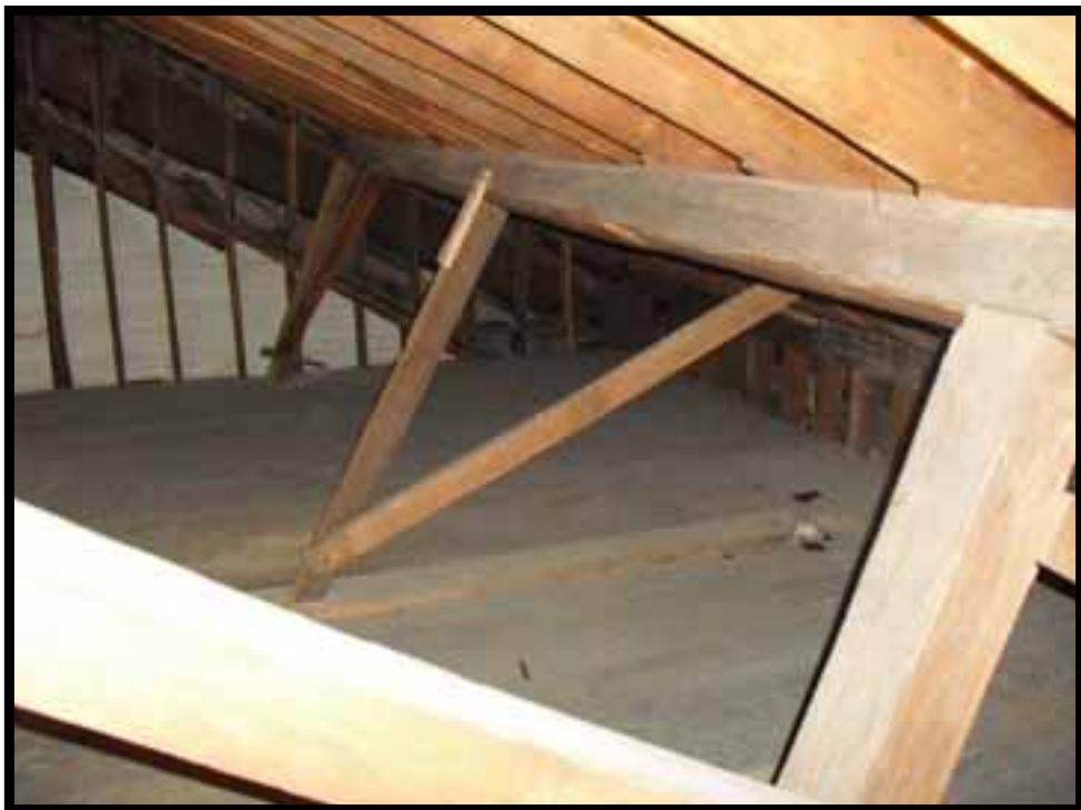
34. LOOKING NORTH WEST AT ROOF FRAMING IN NORTH WEST CORNER OF ATTIC.
