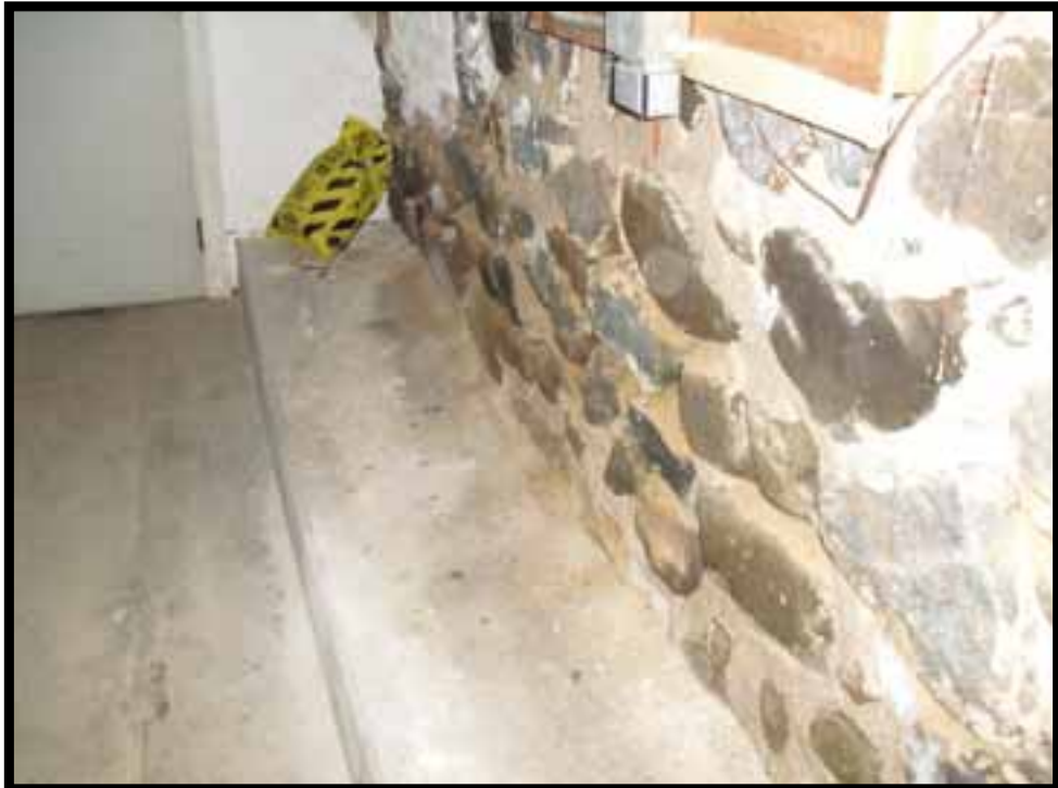
20. WEST WALL OF BASEMENT HAS AREAS OF EXPOSED ORIGINAL MORTAR THAT IS VERY SANDY AND IS FALLING OUT OF THE JOINTS BETWEEN THE STONES.
