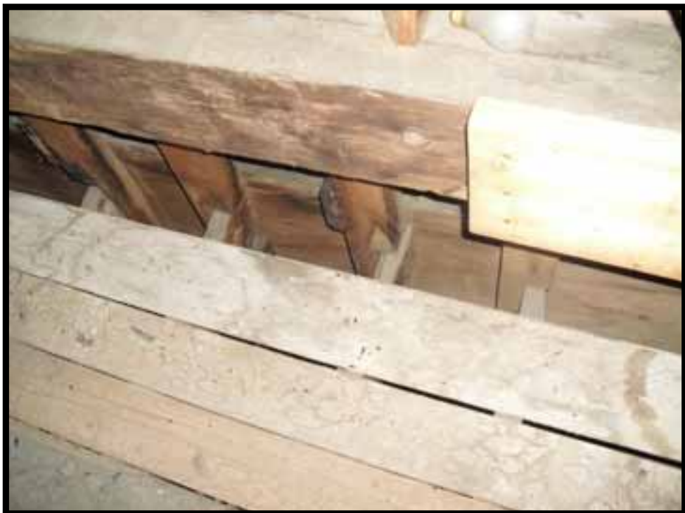
48. SUPPORT OF ATTIC FLOOR JOISTS AT EATS GABLE END WALL.
