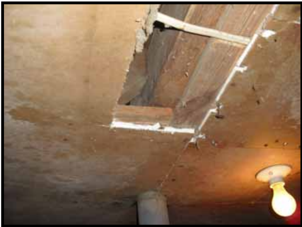
10. CENTRAL TIMBER BEAM IN S-W CORNER BASEMENT ROOM SPANS EAST WEST AND IS SUPPORTED BY PIPE COLUMN AND BRICK PIER. JOISTS MORTISE IN.
