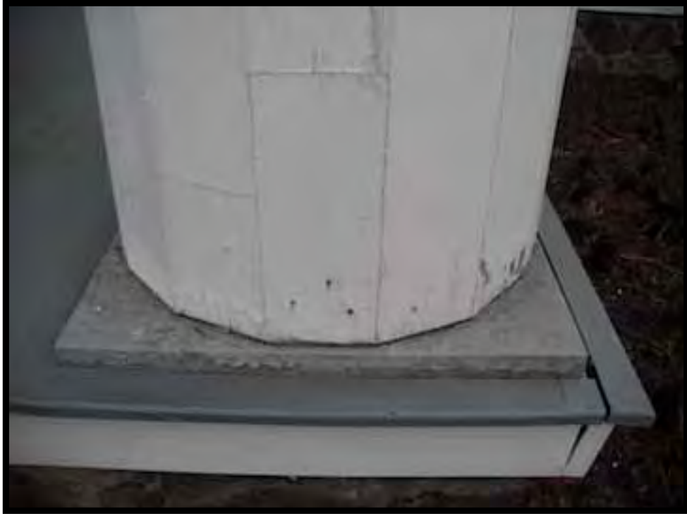
57. BASE OF NORTH EAST PORCH COLUMN.
