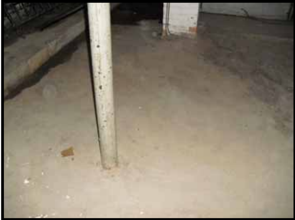
19. COLUMNS SUPPORTING 8X8 TIMBER BEAM SEEN IN PHOTO 18 DISAPPEAR INTO SLAB AND ARE LIKELY SUPPORTED ON FOOTINGS.
