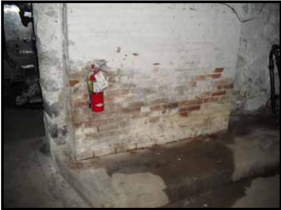
21. WATER LEAKING FROM NORTH WEST CHIMNEY.
