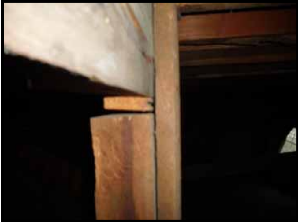
41. POOR CONTACT BETWEEN ROOF PURLIN AND INCLINED COLUMN.
