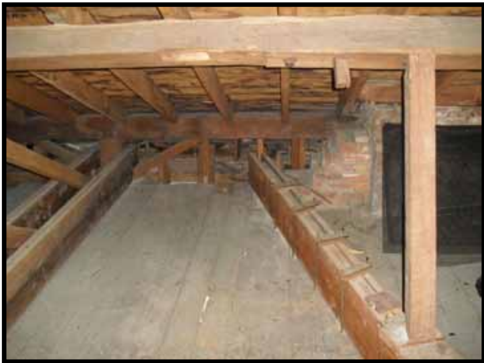
32. LOOKING NORTH. NOTE SCARF JOINT IN TIMBER PURLIN AND NON ORIGINAL BEAMS ABOVE ATTIC FLOOR.
