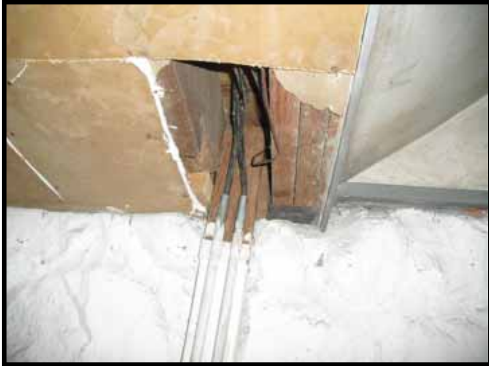
15. NON ORIGINAL (2)2X10 HEADER AT NON ORIGINAL STAIR OPENING FROM FIRST FLOOR TO BASEMENT.
