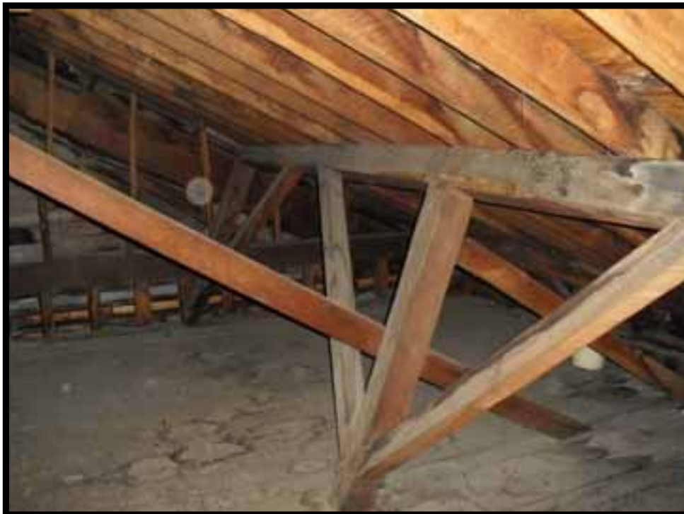
30. LOOKING SOUTH EAST AT ROOF FRAMING IN SOUTH EAST CORNER OF ATTIC.
