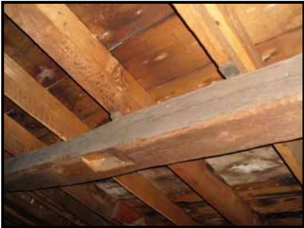
52. ROOF PURLINS APPEARS TO HAVE BEEN RE USED DUE TO JOIST HOLE WITH NO MEMBER FRAMING IN.
