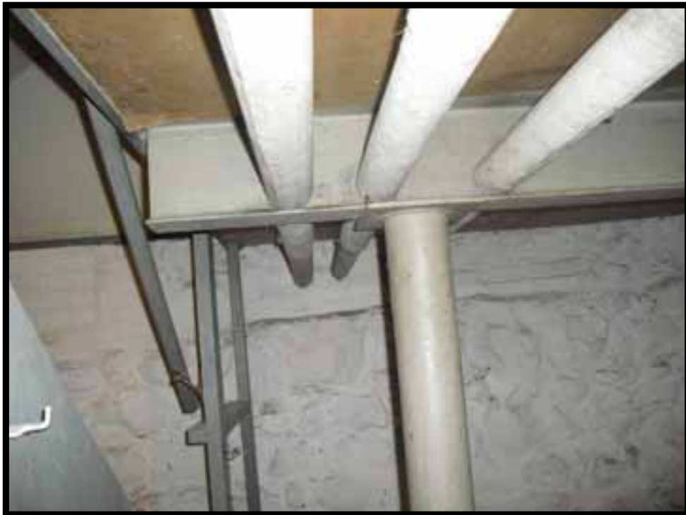
16. NON ORIGINAL I BEAM SUPPORTS JOIST AT EDGE OF ORIGINAL STAIR OPENING TO BASEMENT WHICH IS CURRENTLY FLOORED OVER.
