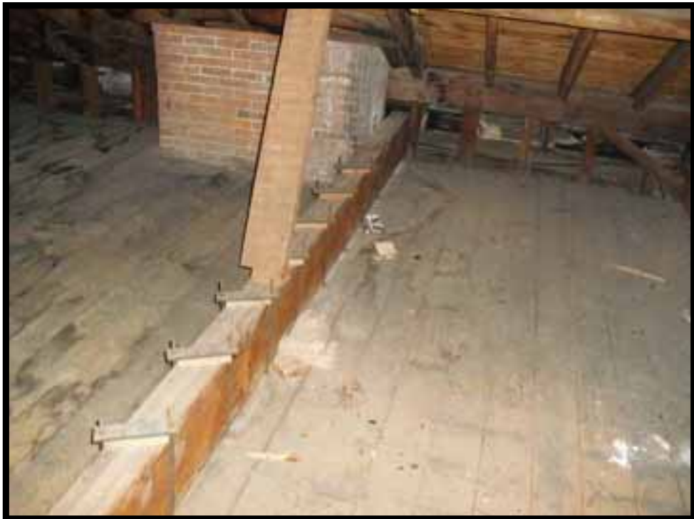
28. NON ORIGINAL BEAM HANGING ATTIC FLOOR AND SUPPORTING SLOPING COLUMN FROM ROOF PURLIN.
