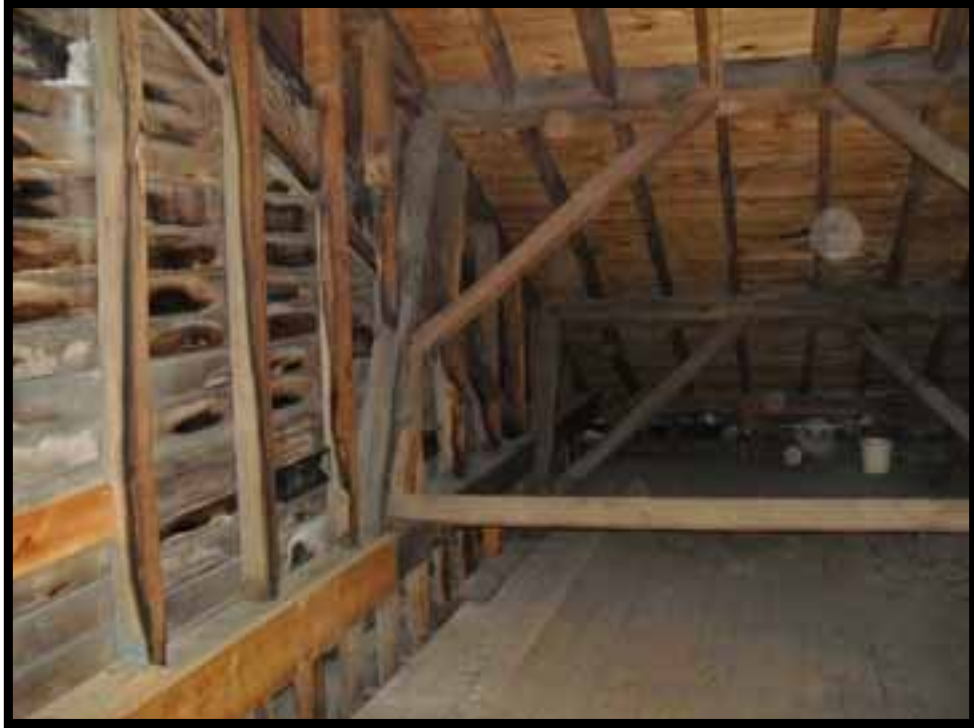
51. ATTIC FLOOR AND ROOF FRAMING LOOKING SOUTH NEAR EAST GABLE END WALL.
